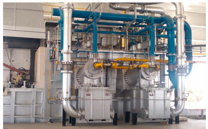
\ Sidewell melter 65 Ton with regenerative burners.
